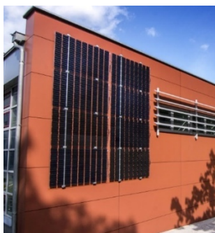
Fig.1. View of the Chemistry C building with BIPV installation
