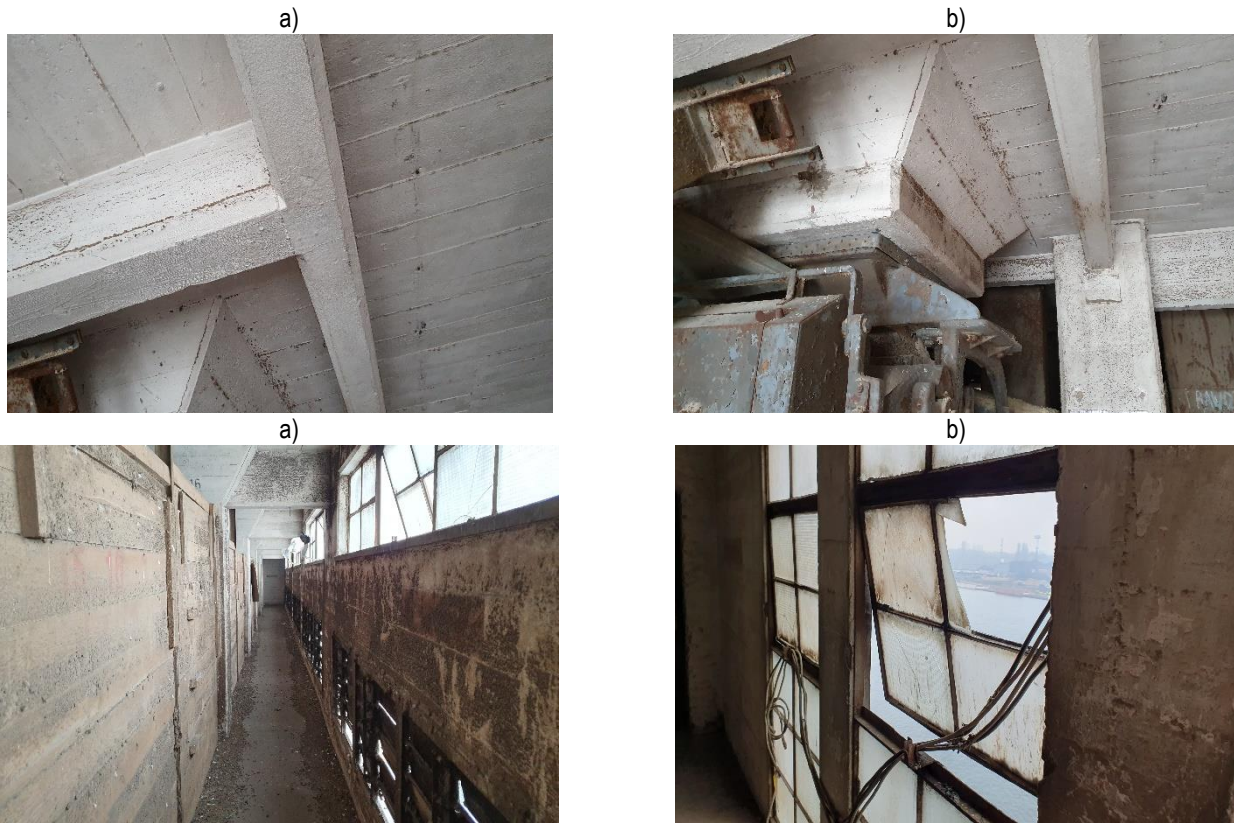
Photo 5: Grain Elevator building - level +5: a) mechanical damage to structural elements, b) equipment for transporting loose materials left inoperative and incomplete, decapitalization of: c) ventilation shutters, d) window joinery
