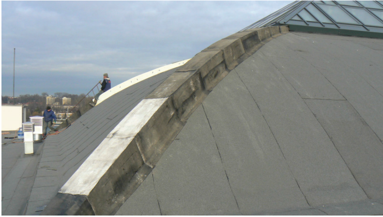
Fig. 18. View of the insulated ribs of the dome of Gdynia Seaport Dome (December 2013)
