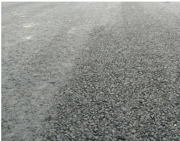
Figure 3. Surface of the lower asphalt base course AC22P. Non-homogenous surface. Road R1S.
