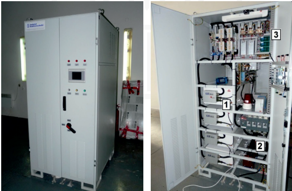
Fig. 5. Supercapacitor energy bank installed in the traction substation Północna in Gdynia; 1 – supercapacitor modules, 2 – DC/DC converter with the controller, 3 – protection modules and filter
