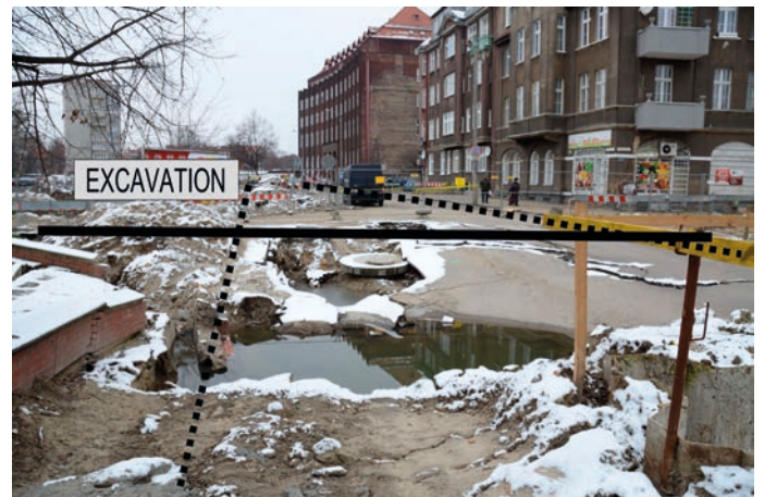
Figure 12. General view of Gdańsk 2013 real-life case of a pipe failure in the vicinity of an unsecured excavation that inspired this study Dotted lines indicate road edges while solid line indicates the axis of the pipeline
