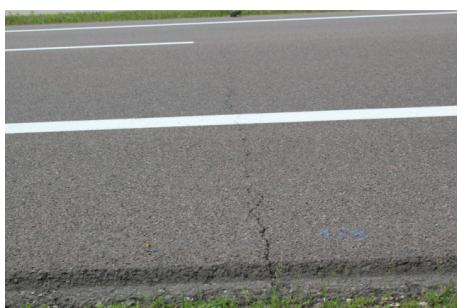
Figure 2. Not repaired low-temperature crack.
