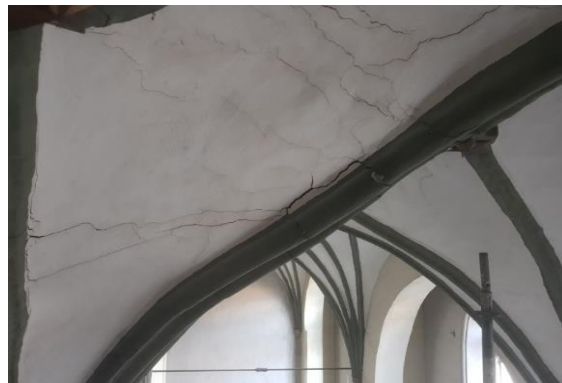
Photo 3. Damage to the diagonal ribs (deformations, scratches and cracks) of the southern aisle of the Basilica of St. Nicholas in Gdańsk ( photo by T. Majewski )
