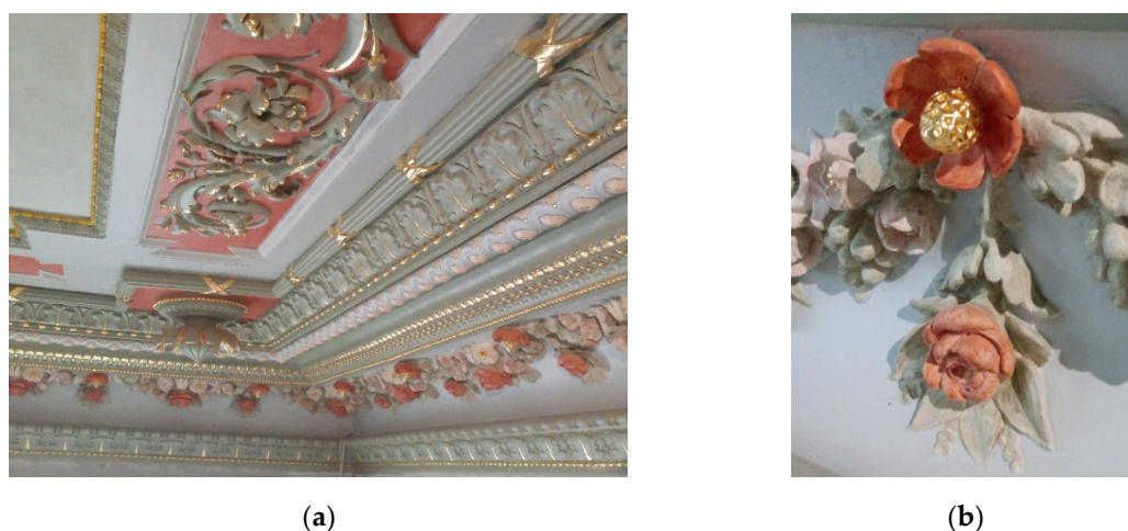
Figure 2. Stucco renovation on the ceiling: (a) partial view on the ceiling; (b) view of the gilded floral detail.
