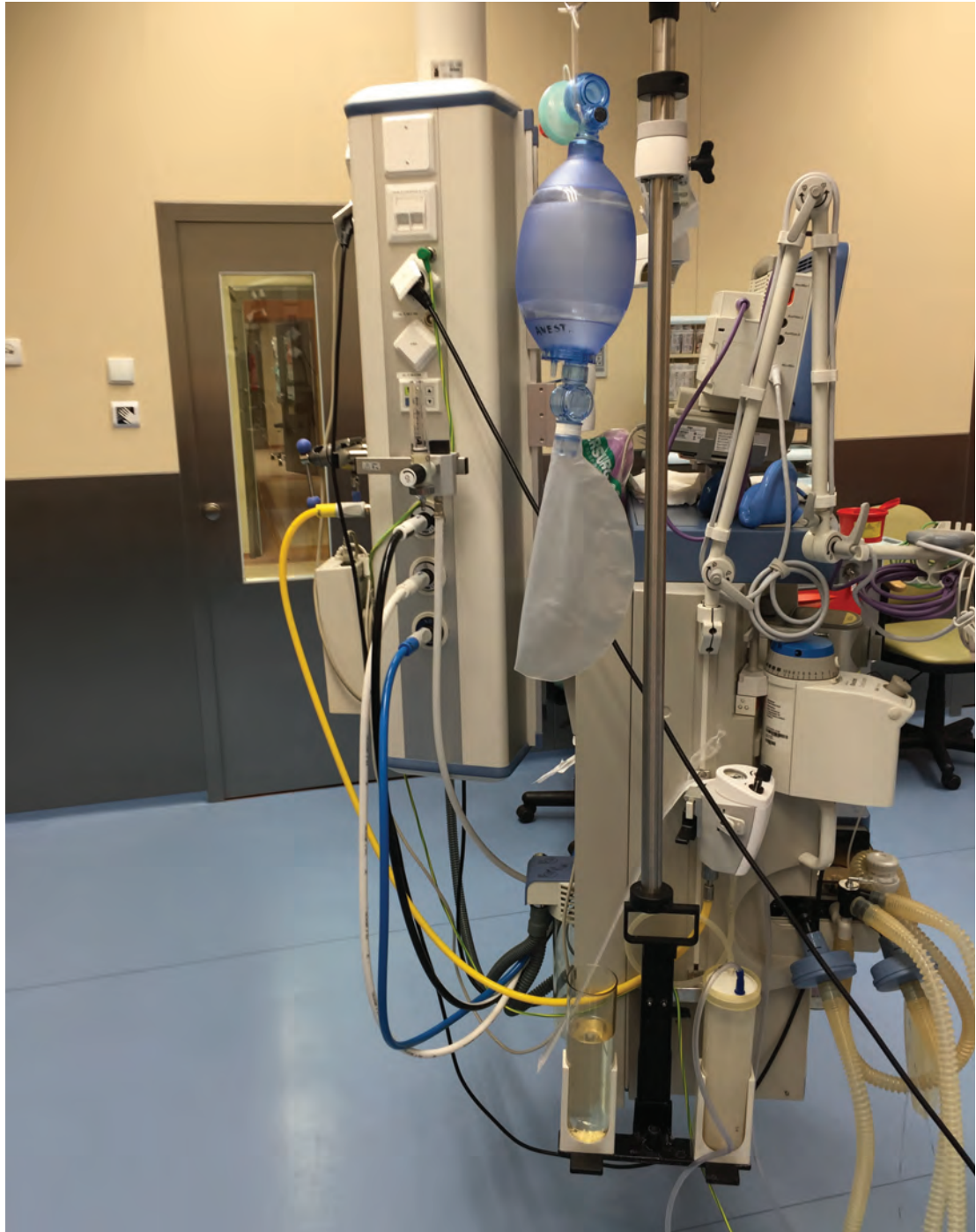
Photograph 6.2.3.6 The equipment in an operating theatre (a possibility of suspending some elements on a column facilitates disinfection of the floor); photographed by the Author, 2016
