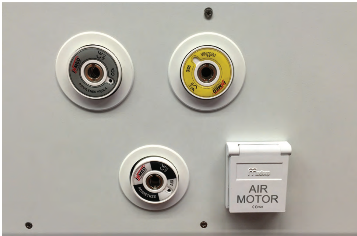
Photograph 6.2.3 Terminal units for medical gas pipeline systems (technical infrastructure may become a hospital-acquired infection source); photographed by the Author, 2016
