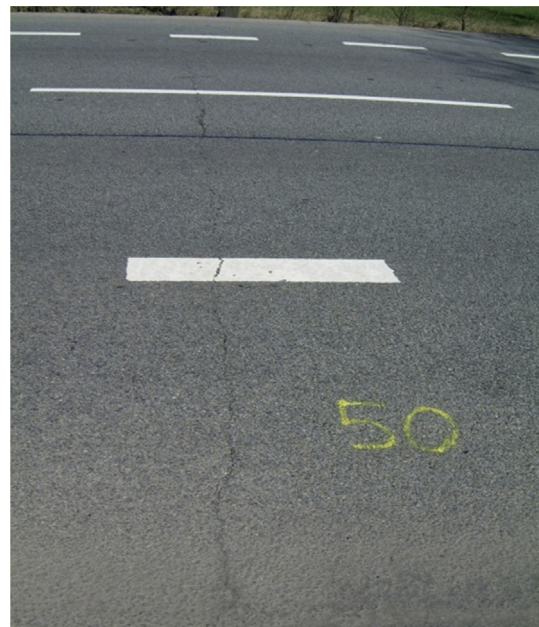
Fig. 5 – Transverse crack in pavement with an MCE base.
