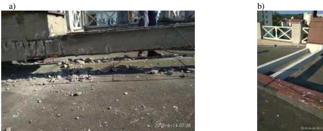
Photo 11. Reinforced concrete, monolithic beams of the grate supporting the cross from the west elevation (along 3 Maja Street) - condition: a) before, b) after renovation (street names as of 2023) (photo by Maciej Niedostatkiwicz)
