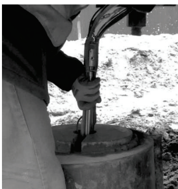
Figure 4. VWSG Model 1300 A-9 installation in a pile.
