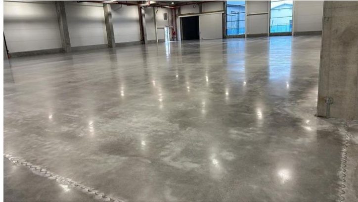
Fig.7. Concrete industrial floor (Example 2) after regeneration by polishing and impregnation process: a), b) view of pavement treatment in the area of structural expansion joints
