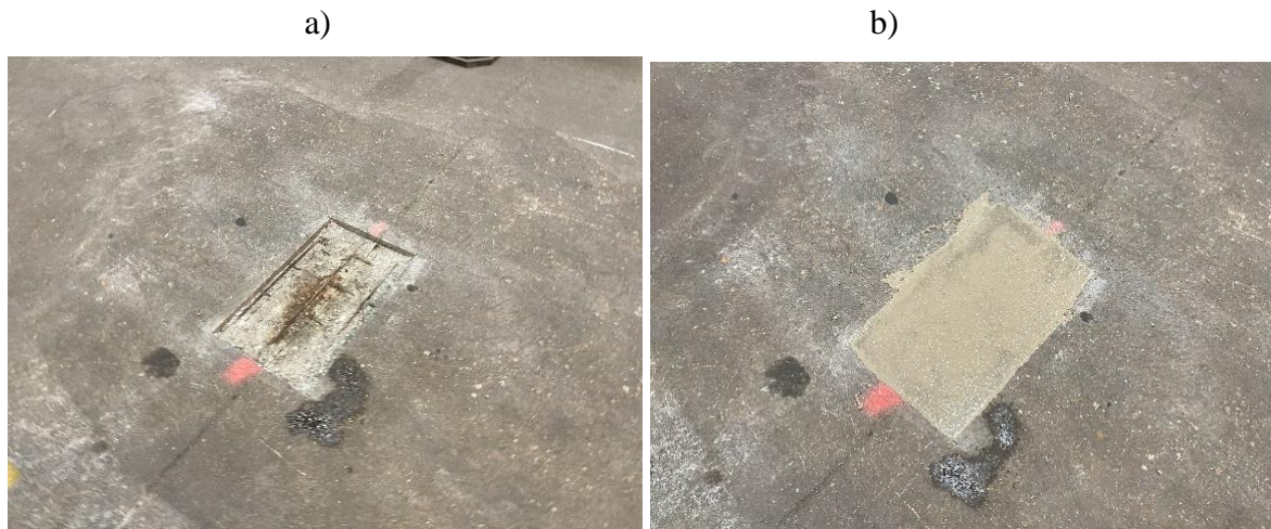
Fig.4. Concrete industrial floor (Example 1) filling of defects: a), preparation of work area b) filling of work area with repair compound
