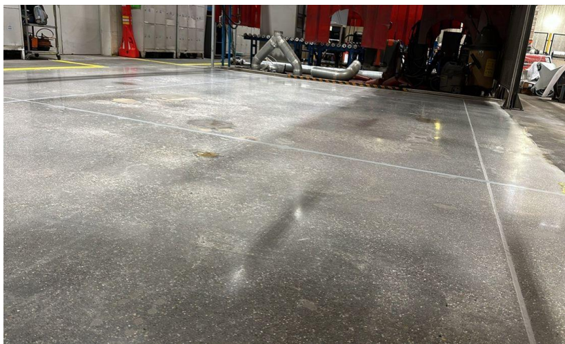
Fig.5. Concrete industrial floor (Example 1) after repair: a) view of shiny surface and expansion joint fillings, b), c) view of filled cavities and filled expansion joints
