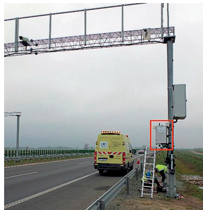
Fig. 30.1. Measuring station (marked with a red rectangle) mounted on the gantry pillar
