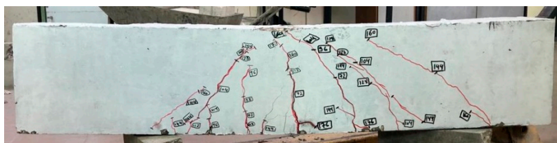
Figure 18. Crack pattern for beam PS-0.
