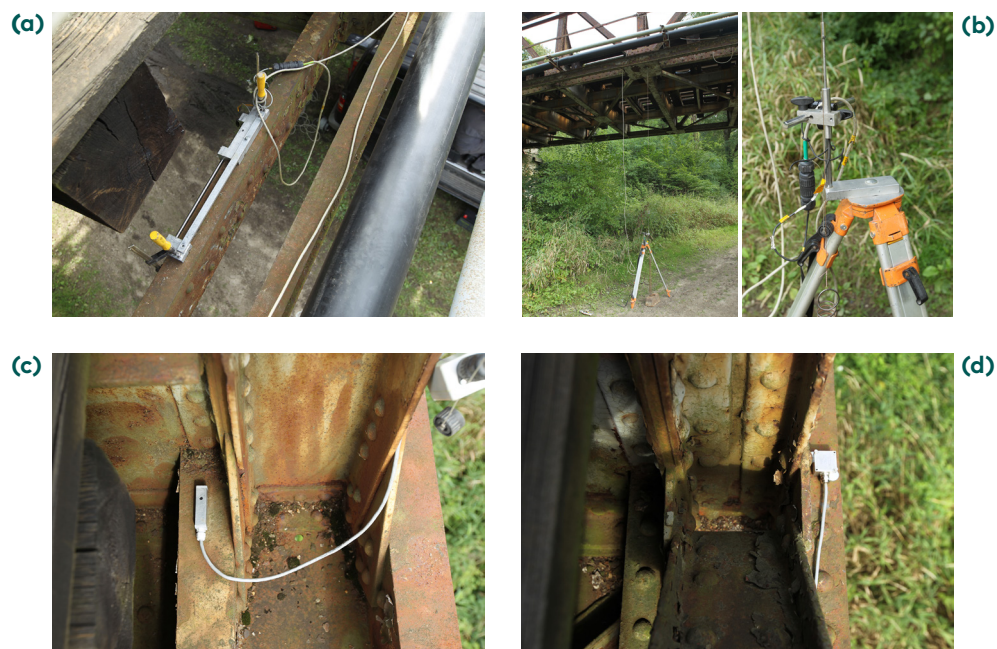
Figure 9. View on chosen measurement points: (a) – Strain measurement point; (b) – Vertical displacement measurement point; (c), (d) – Acceleration measurement points
