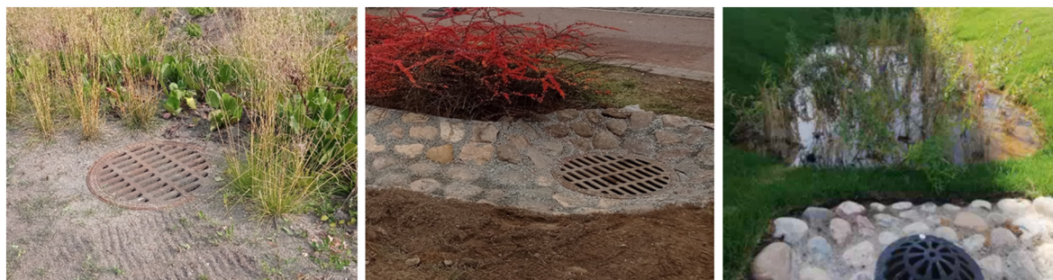
Fig. 8. Emergency overflow directed to the storm water drainage system.
