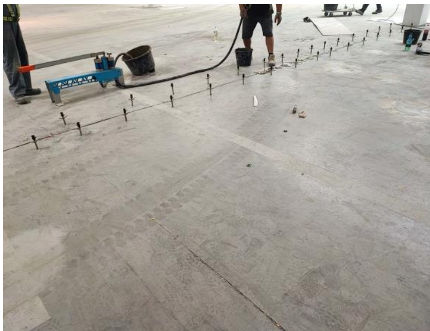
Fig. 16. Concrete industrial floor (Example 4) during repair: installation of packers and feeding of cement injection with a pump [38]
