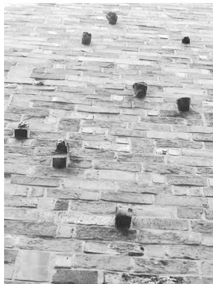
Photo 5. Black “pimples” on the façade of Helmholtzstrasse multifamily house
