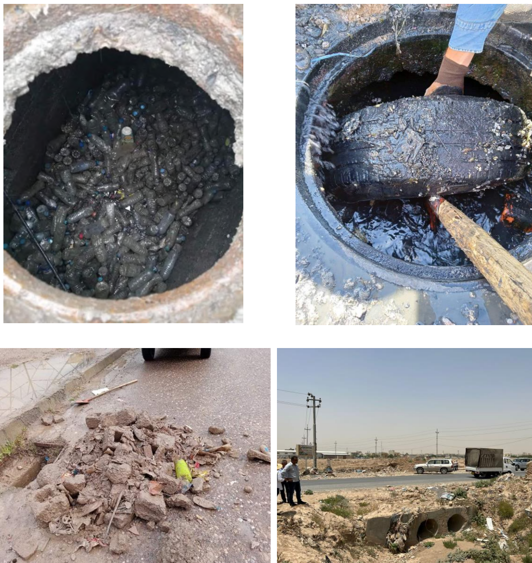
Figure 49. Debris and waste accumulation inside culverts, sewer pipes, and natural streams.
