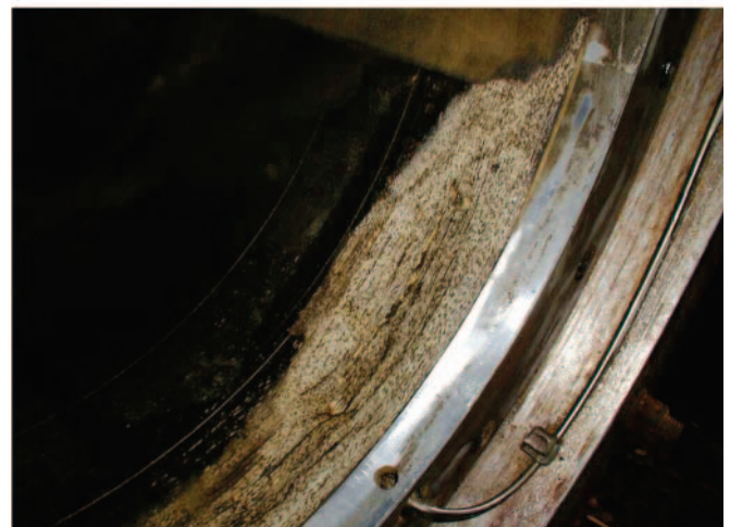
Fig. 3. Damage of a composite bush, resulting from edge thrust resulting from skew position of shaft axis (up); during repair the damaged edge was grinded to avoid cracks and delamination of the composite (down)
