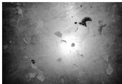
Fot. 2. Uszkodzona posadzka parkingowa na skutek korozji [Fot. Autorki] Photo 2. Damaged floor parking due to corrosion [Phot. Authors]
